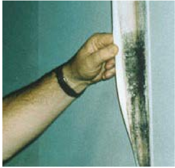
Hidden mold growing behind wallpaper.
