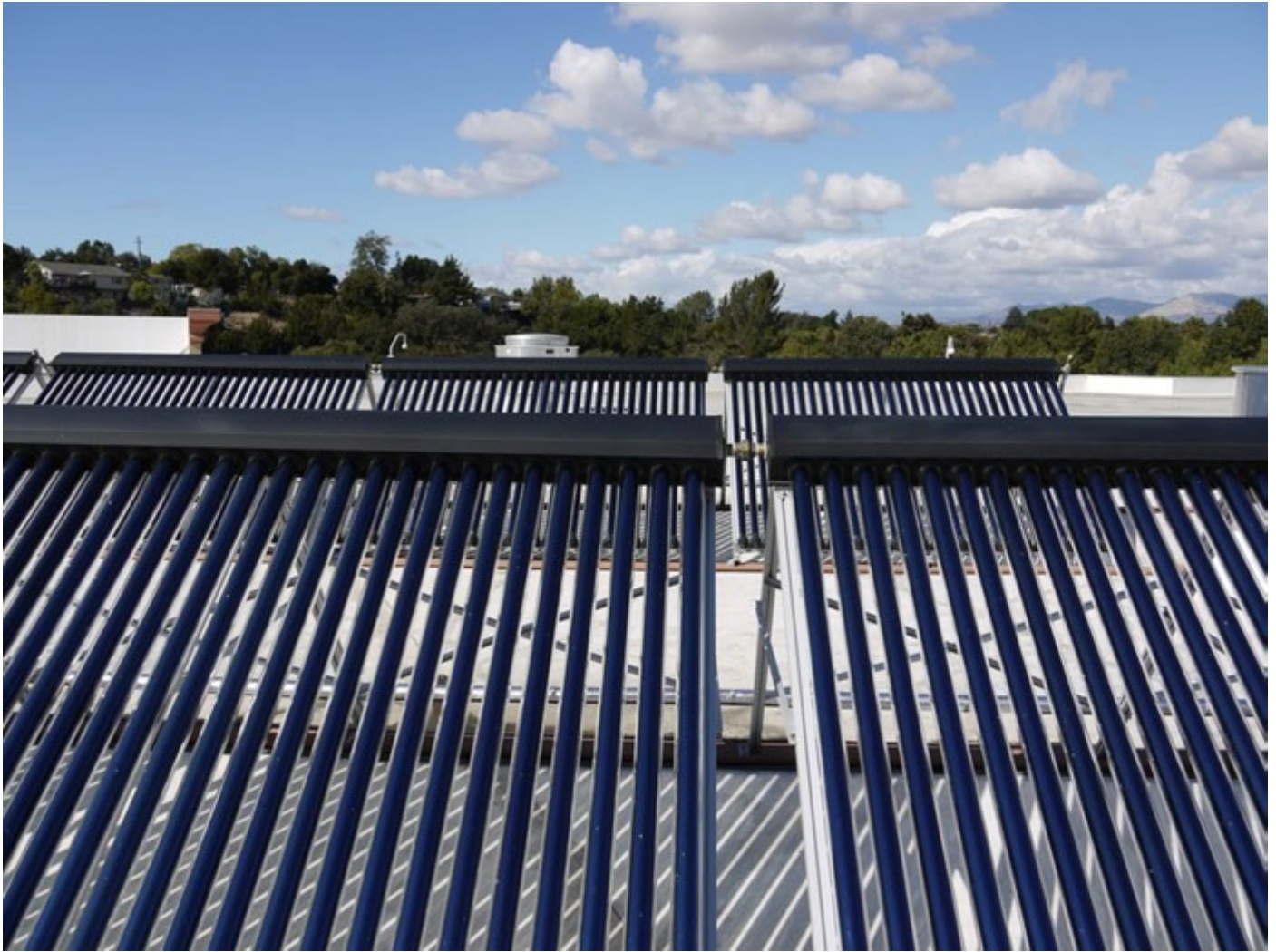
Santa Ynez Band of Chumash Indians in California: Solar thermal system on top of Chumash Casino Resort
